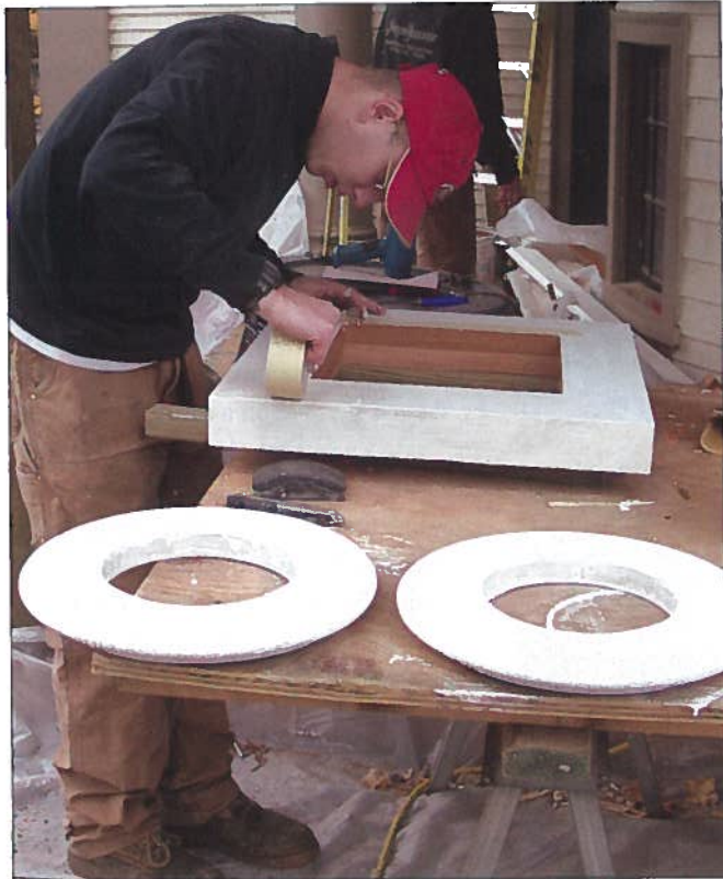
Decay below the column shafts was extensive. The plinths and bases had to be completely rebuilt out of mahogany.
