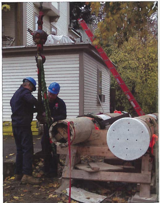
The columns, waiting for reinstallation, show a rebuilt bottom with vent holes, next to a top, still in good condition.
